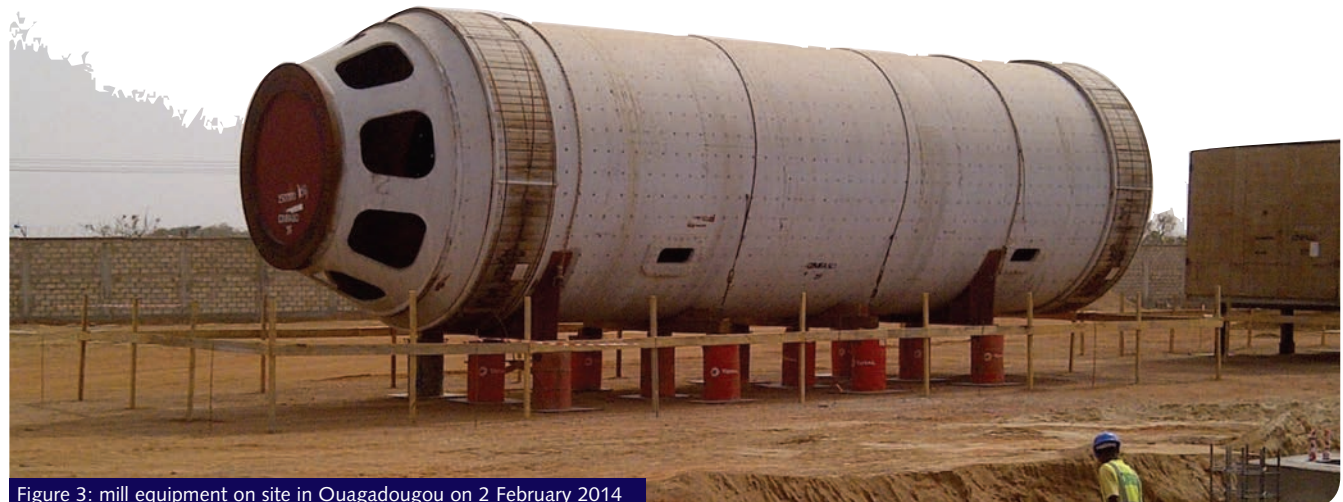
Figure 3: mill equipment on site in Ouagadougou on 2 February 2014
