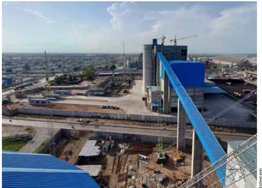
6 All material conveyors are mounted in a closed gallery to ensure dust-free transport
